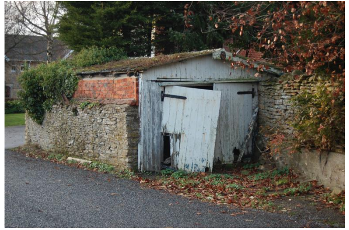
Derelict garage in Dovecote Lane
